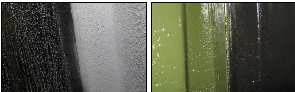
Figure 7. Side By Side Full Scale Corroded Sheet Pile Coating Trial Examples
