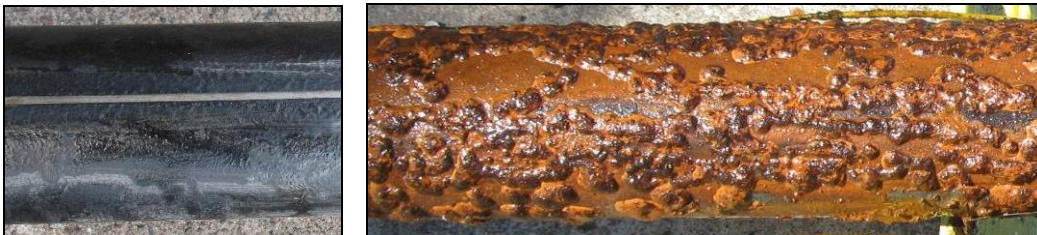
Figure 9. Pipe Samples With and Without Cathodic Protection
