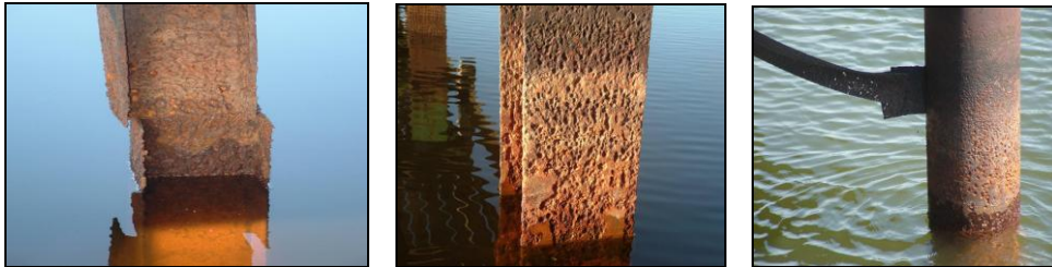
Figure 10. Other Harbors With Lake Superior Corrosion Examples
