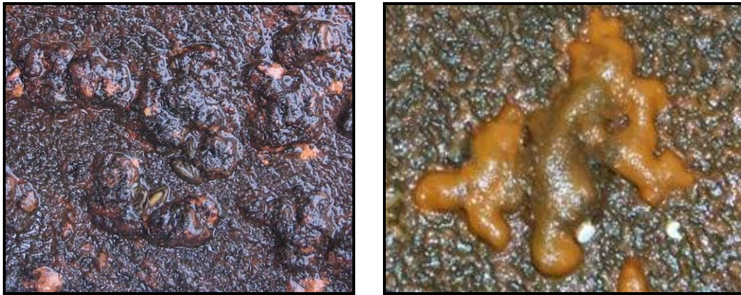
Figure 3. Tubercle Growths Associated With Corrosion
